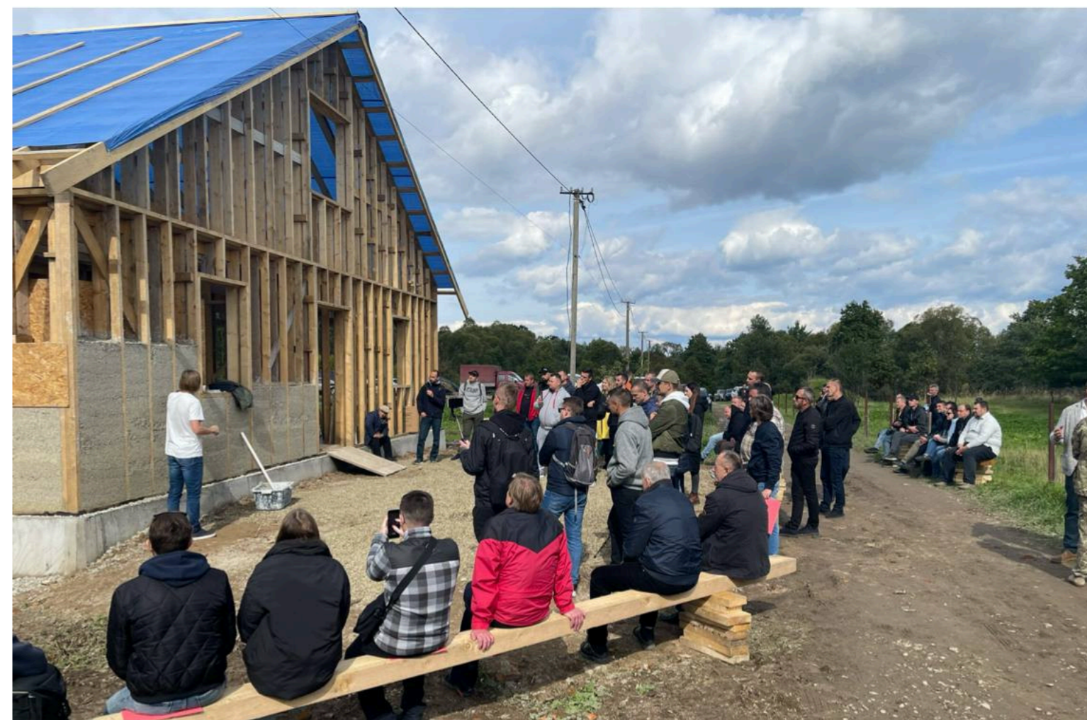
Construction of eco-friendly housing for refugees using Hempire TM (hempcrete) technology while training internally displaced persons in this technology.
