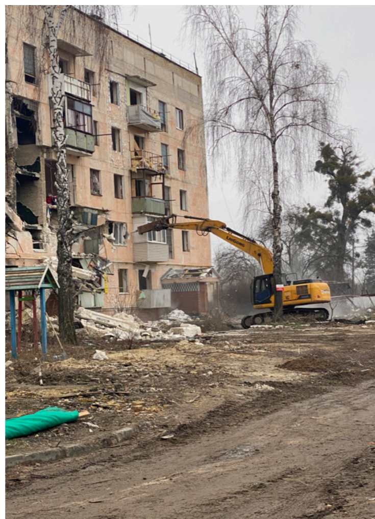
Neo-Eco Ukraine is dismantling a damaged high-rise building in Gostomel. Photo provided by the company.
